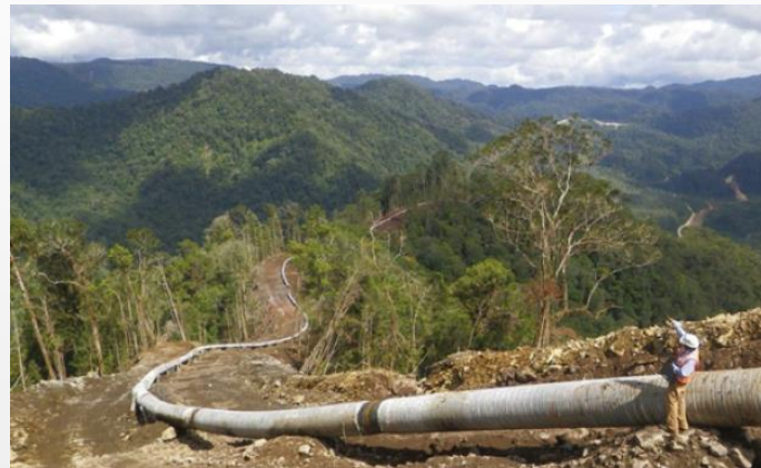
Landslide-induced pipeline failure (Georgia/Caucasus) – July 2020
