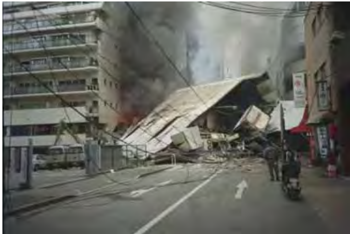
FIGURE 9: COMPLETELY DESTROYED CONCRETE FRAME OFFICE BUILDING, GREAT HANSHIN-AWAJI (KOBÉ) EARTHQUAKE, JAN 1995 PHOTO CREDIT: DR. ROGER HUTCHISON, NGDC, NOAA
